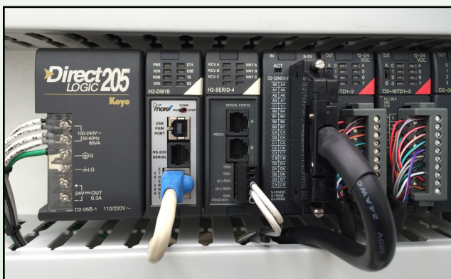
PLC Hardware with I/O Module
