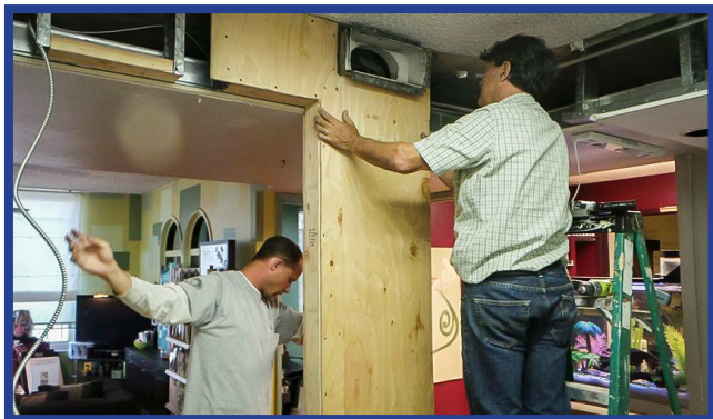
Once again Francie is expanding the "Final Cut Hair Studio & Tranquility Lounge" by taking over a small office that was recently vacated. Of course that meant father and son team, Ed & Nathan Riel, were called into action. Nathan, the new family electrician, relocated a power panel, added some lights and reworked the power outlets for the new area. While Ed, of course, did everything else. Be sure to drop by soon to see the latest expansion.
